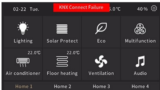
KNX connect failure
